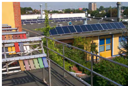
Photo-voltaic and solar heat installations
